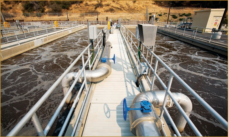
FIGURE 7.1 Water is purified at the Hill Canyon Wastewater Treatment Plant in Camarillo, California.
